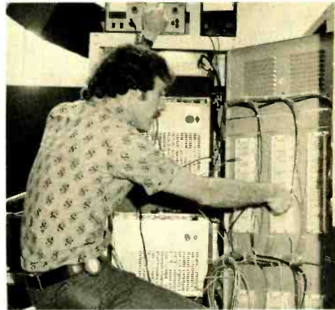
Tracing connections on back of production control studio
