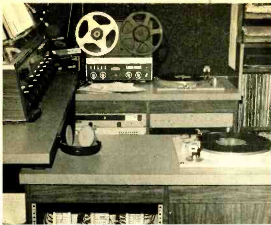
FM Master Control showing Telco blocks
