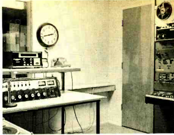
Master control room for the station.
