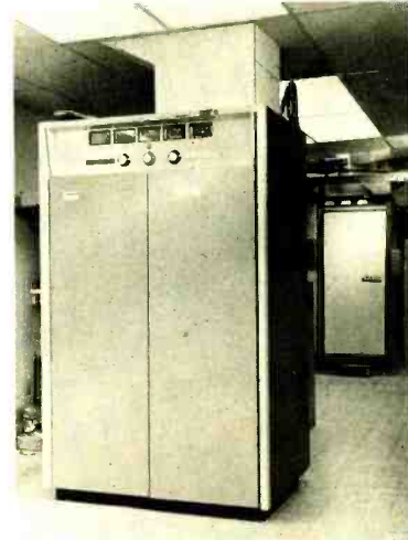
FM transmitter in foreground. AM at rear.
