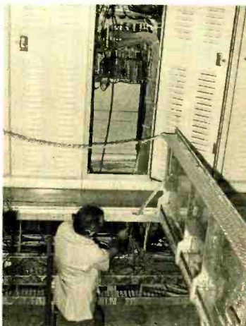
All wiring is dropped straight down into trap located in cable basement. 24 x 20 AFV distribution switcher is shown in rack above.
