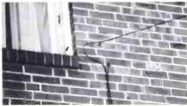
A fatigue loop is also put in drop cable at house attachment.
