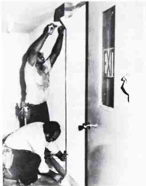
Vertical risers are installed between floors in fire stairwells. Aluminum ducts conceal the cable.
