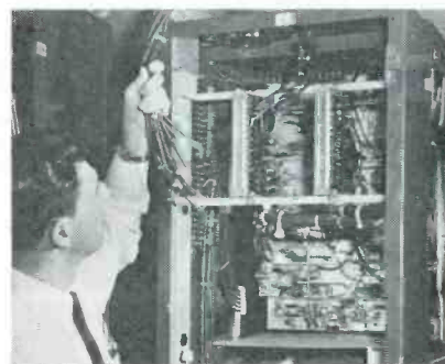
Joseph Caspar, WOR-TV Maintenance Engineer, at the rear of one of the 6 identical camera control racks. Cables are fed into the cabinet through holes in the top and connections are made to the connector blocks.
