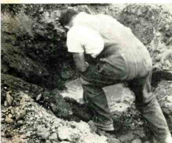
Some holes may end up like this. This water-filled expanse started out like the others; then the auger hit a 6" water main.
