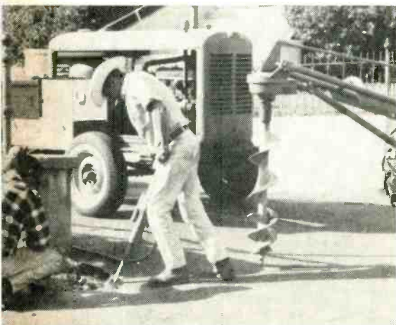
Approximately 5% of the Valley-Vision holes dug in Jackson required the services of a jackhammer. This pole, located at the end of a concrete pier, had to go through 18" of concrete.
