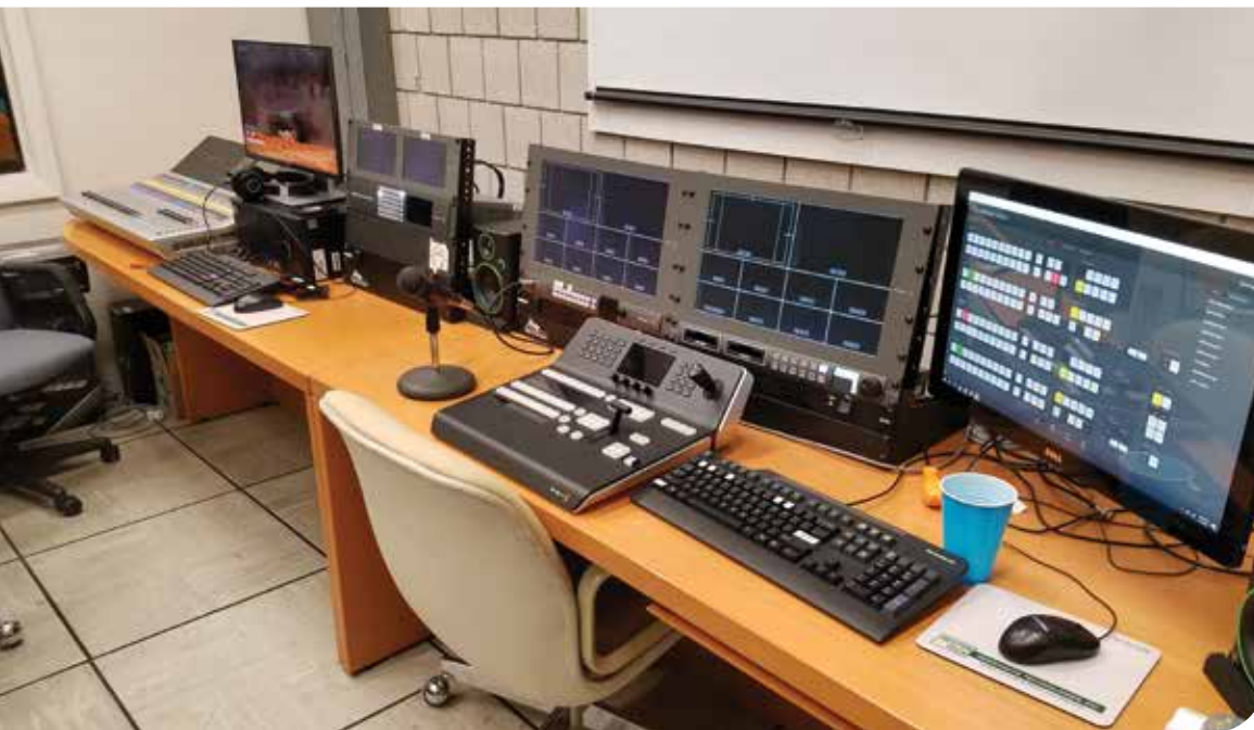
The control room Michael built for Wilton Public Schools.
