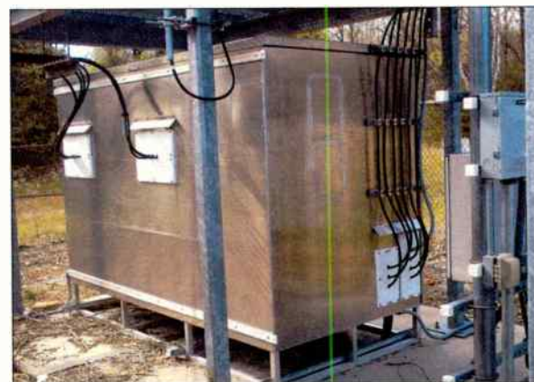
Box with detuning coils for antennas on AM tower.
