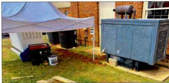
Portable generator under tent.
