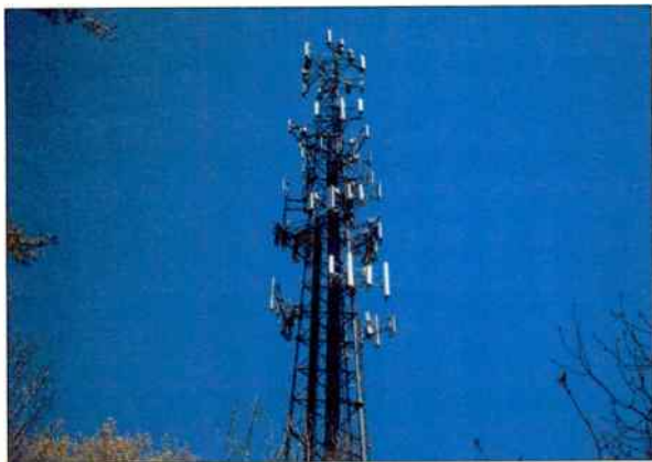
A Very Busy Cell Tower
