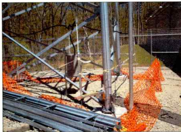
A Detuned Communications Tower
