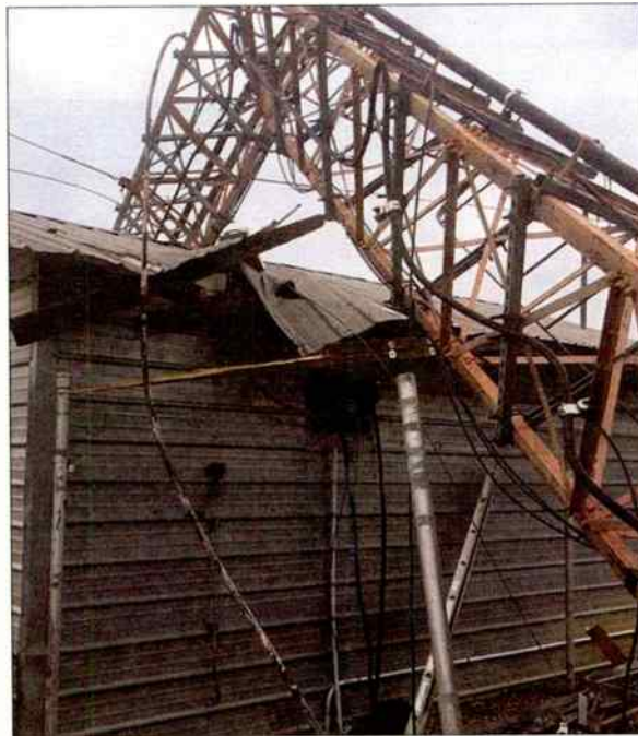
Tower folded over tenant building.
