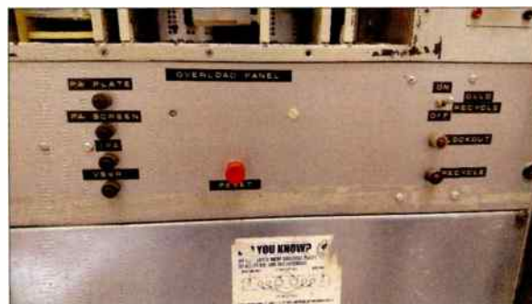
Overload Indicator Panel
