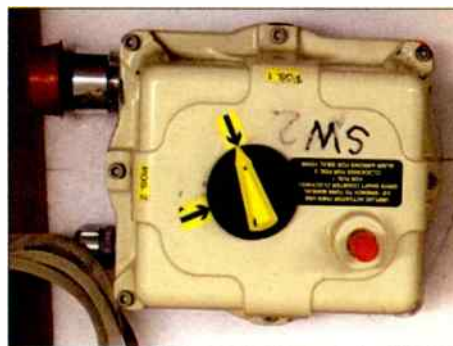
Figure 3. The damaged motor assembly and direction indicator. This whole assembly was replaced by the manufacturer.
