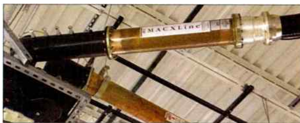
Figure 7. The section as installed between the RF switch and spare antenna coax.
