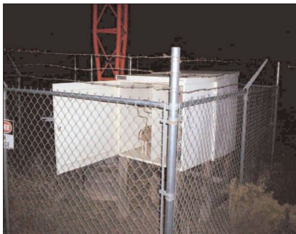
This ATU opened the door to problems.
