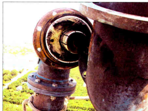
When lightning strikes are not controlled, damage occurs, including hidden damage inside the connectors.
