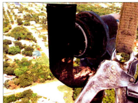
This transmission line shows the effects of a lightning strike.
