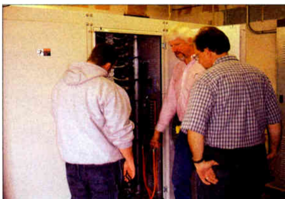
The author explains the power distribution in a new transmitter to apprentice Loren Denison, while Citadel Director of Engineering Martin Stabbert observes.
