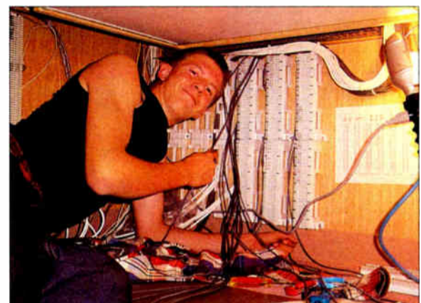
Apprentice Luke Babcock learns to dress console cables to the punch blocks.
