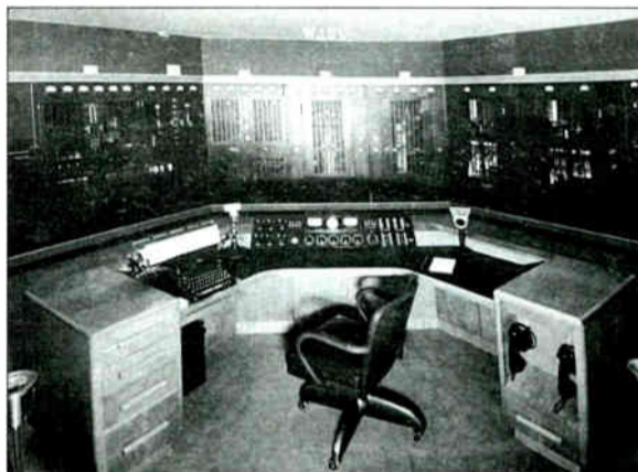
The Western Electric 407A was installed in 1941.
