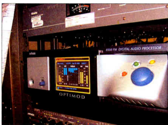
The Optimod 8500 in the WUVT rack.
