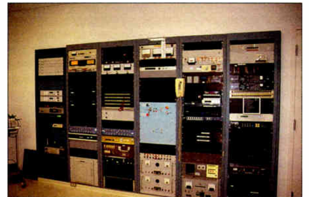
The audio and control racks give evidence of the continuous upgrading that has gone on at WBBM over the years.
