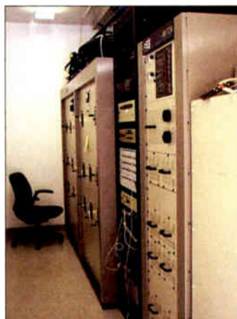
The completed installation in the transmitter building.
