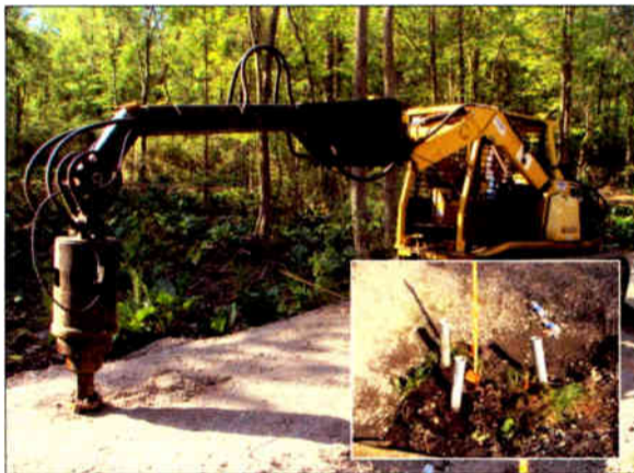
The helical anchors provided the support for the tower foundations and anchors.
