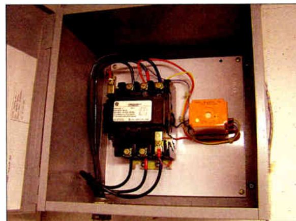
The contactor and Phase Loss module mount inside a 12 x 12 x 6" Hoffman enclosure.
