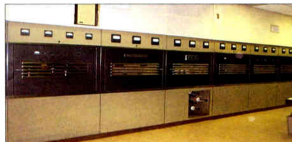
The 50HG1 installed at KEX, Portland, OR.
