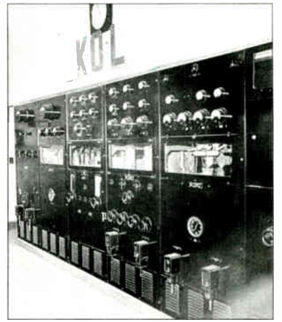
Westinghouse made this RCA branded 5 kW transmitter.
