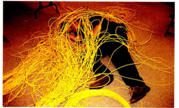
When dealing with a large pile of wires, resistance might be futile.
