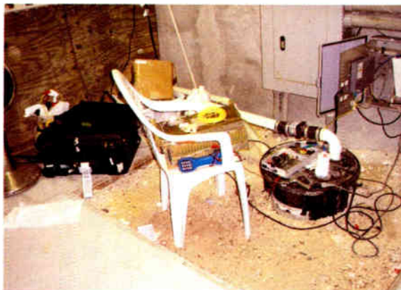
A plastic chair was all that stood between the telco equipment and spark city.
