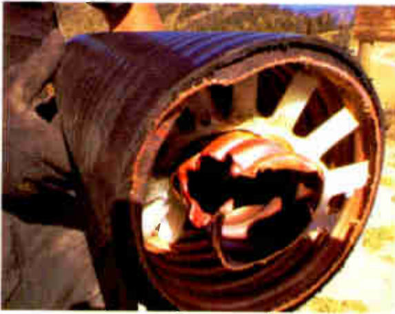
Water in the line plus high power equals bad coax.
