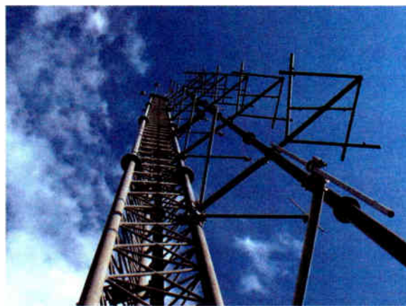
Jampro JHPC-8 antenna on a frequency-matched tower section.
