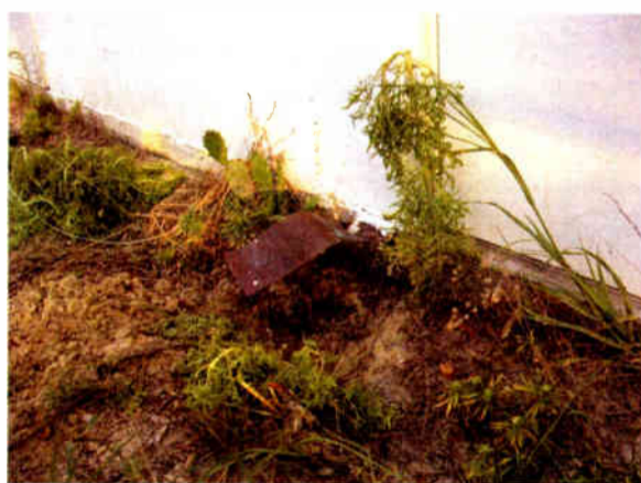
The contractor "forgot" to finish grounding. A little digging revealed several useless ground straps.
