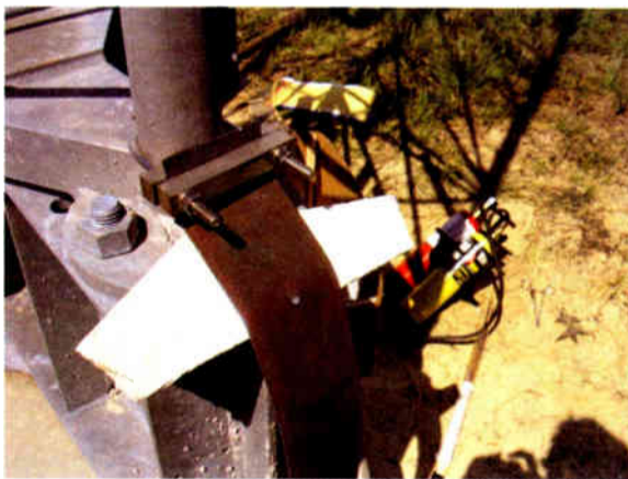
An impressive looking ground clamp, but it really did not work all that well.
