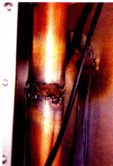
This ex-filter was not going to transfer power very well.
