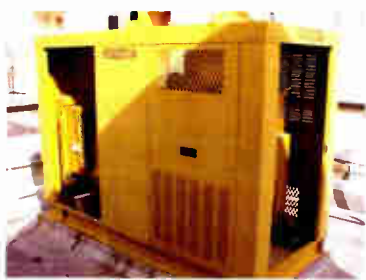
The Generator sitting on the roof.
