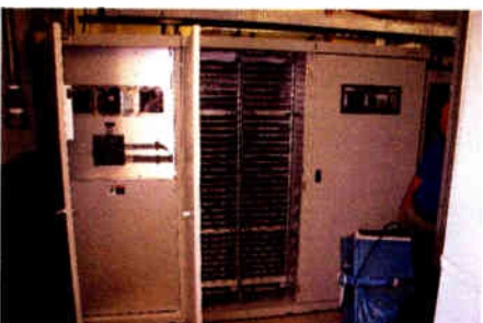
KMOX' new Harris Destiny during installation.
