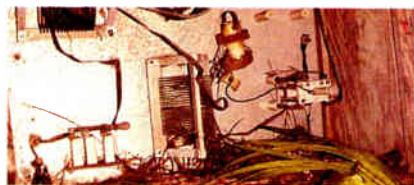
This ATU even has some illegal “tenants.”
