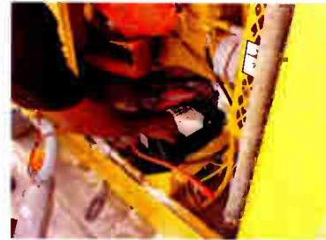
Installing a new battery. This one has caps and will need to be refilled, but perhaps it will not explode as easily.
