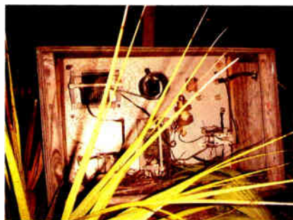
This is an operating ATU!
