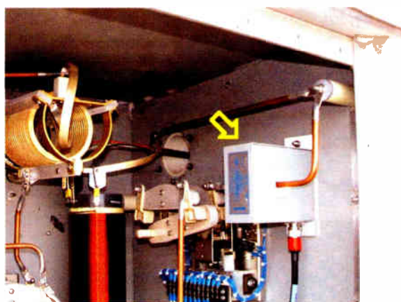
Typical toroidal current transformer installation.
