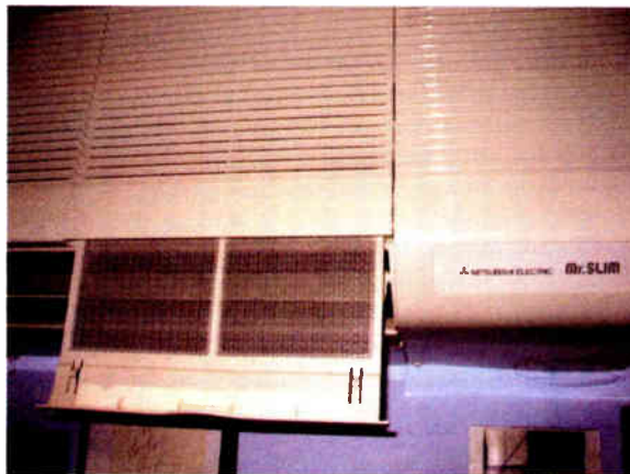
AC units run much better with clean filters.
