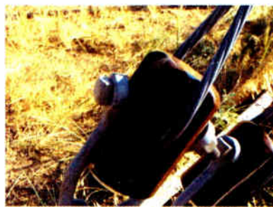
A guy wire insulator that should be replaced.
