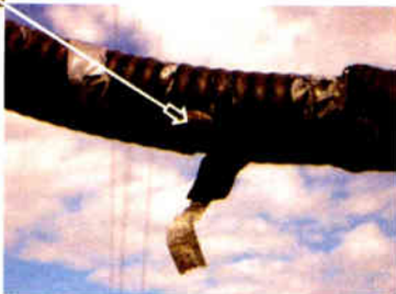
Notice the duct tape "latch" for the weephole.
