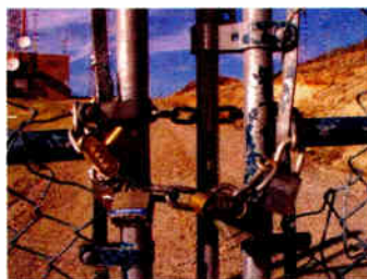
The "Chain O' Locks" One misplaced lock can prevent access in an emergency.
