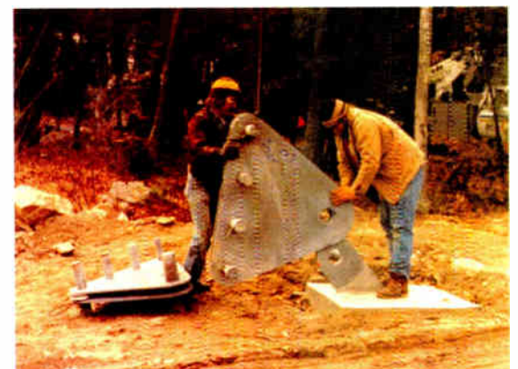
Rigging work is tough and demanding even on the ground. Two pros manhandle a tall tower anchor fanner plate adapter into place to be “pinned.”
