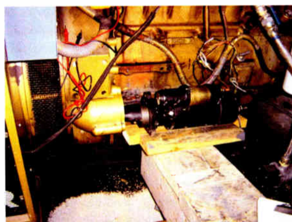
New starter being set in place with "car ramp" to hold it while mounting.
