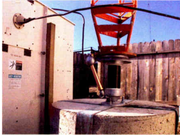
Our nice new insulator holds the tower up.
