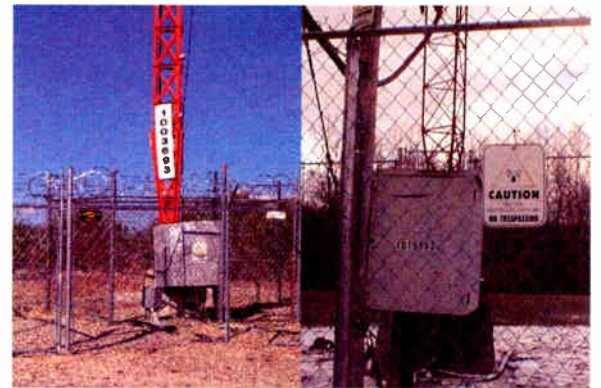
ASR sign at tower base. ASR on ATU box.
