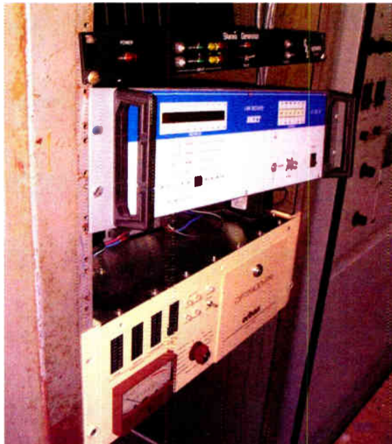
Rack equipment that had fallen out when rack screws sheared during the quake.
