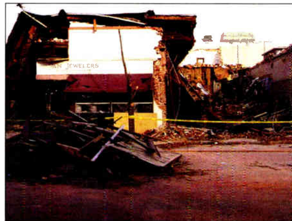
When the roof slid off there was nothing left to keep the walls of the adjoining building apart. The result was they collapsed into themselves.
