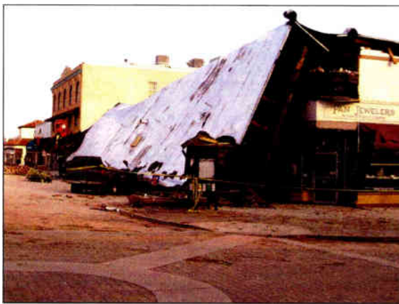
The "Acorn Building" Paso Robles, CA where two persons died during the quake.
