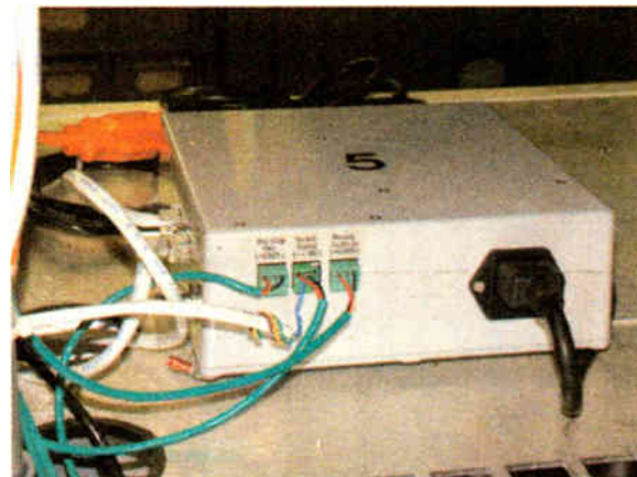
The iBiquity interface box lives on top of the DX-50 transmitter. It converts the RF signal from the Cat-5 cable to a BNC connection, and converts the audio signal to a Phoenix type terminal block. As an added feature, it controls a relay in the transmitter which will switch the transmitter to its internal oscillator should the IBOC exciter fail.
