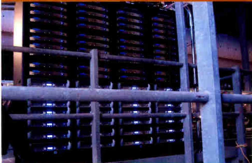
Crown International CT Series and I-Tech amplifiers on catwalk platform.
