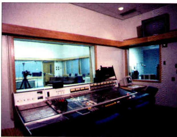
Master control room. Shown here is the vintage Ward Beck M2484 console and views into the audio tracking room and the FM master room.
