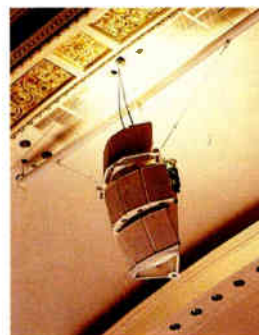
Carnegie Hall A coherent array of UPA-1A loudspeakers, supplemented by MSL-3s and 650-R2 subwoofers (not pictured), is permanently installed for live performance reinforcement.
