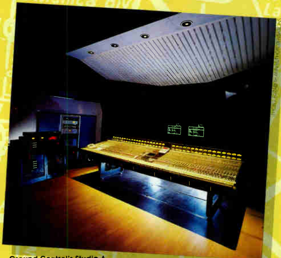
Ground Control's Studio A control room features a 60-input SSL SL 4000 E-Series with Total Recall automation, two Studer A800 analog 24-tracks, Studer A820 analog 2-tracks, a Mitsubishi X-850 PD-Format digital 32-track, a Timeline Lynx time code synchronization system, plus TAD TSM-1 monitors powered by Studer and Perreaux amplifiers.
