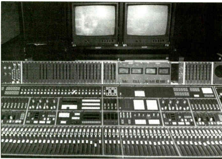
Digitally assignable Calrec console installed in BBC Master sound control vehicle.
