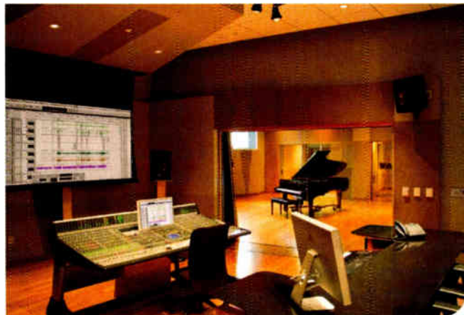
Sweetwater Productions' Studio A includes a C7 grand piano with MIDI in addition to Pro Tools HD3 and a Digidesign ICON with D-Control.
