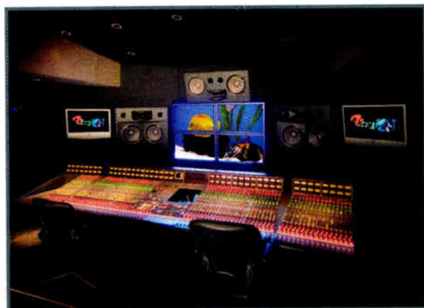
The monitor wall was rebuilt to complement the SSL 9000 J installation; the four plasma screens have been dubbed "the fish tank."
