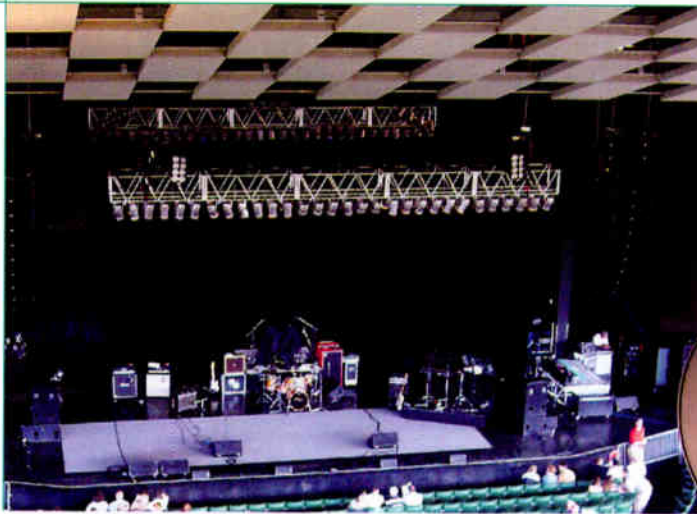
MBI Products' Lapidary Panels installed in DTE Energy Music Theatre's ceiling help reduce reflections. Also shown is the venue's new EAW KF760/761 line array.
