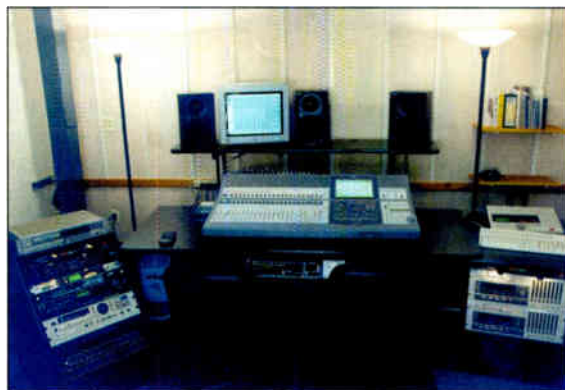
Studio B was recently remodeled, including installation of a Sony DMX-R100 console and Mackie HR-824 surround monitoring.
