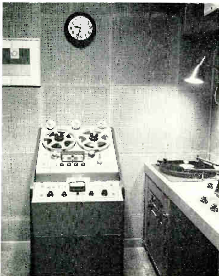
Fig. 4. The tape recording and playback machine and the turntable are installed in the air-conditioned control room at the left of the window
