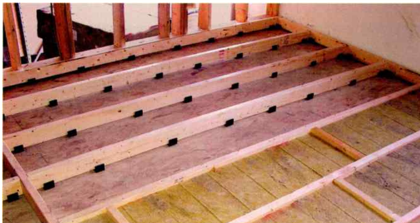
Fig. 2: The construction process. Note how the isolators separate the floor support boards from the "real" floor.
