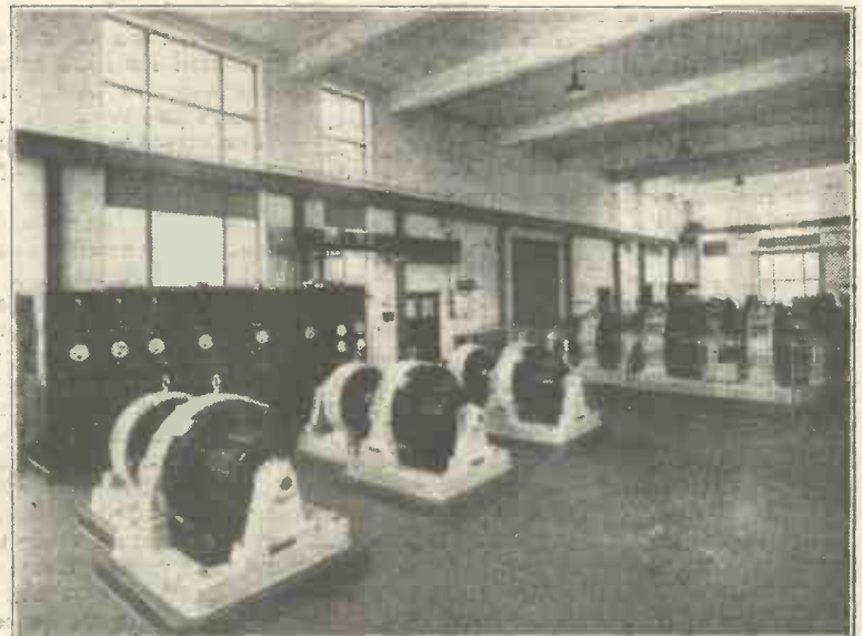
The motor-generator room, showing 3 L.T. generators and 3 12,000-volt H.T. generators
