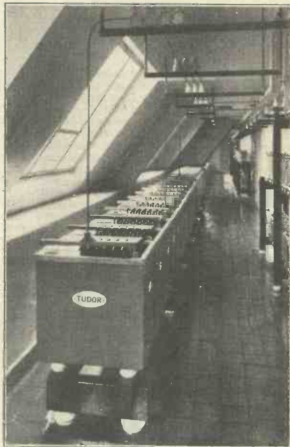
Storage batteries (24-volt, 1,000 ampère-hours) for operating control room relays
