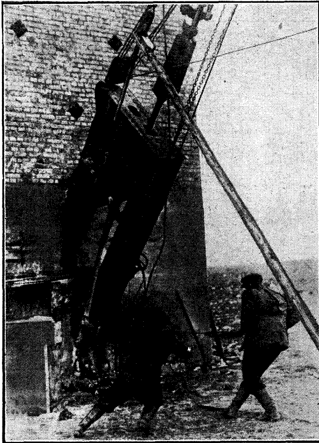
One of the more serious objections to the long-wave station is to be found in the very elaborate engineering work involved by the large aeriels.
