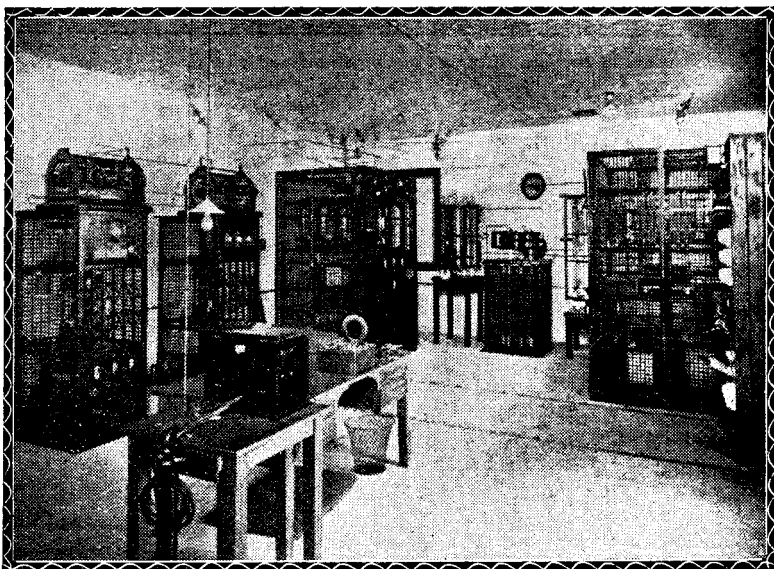
The transmitting equipment at Braybrook from where the programmes from 3LO, Melbourne, are sent out.
