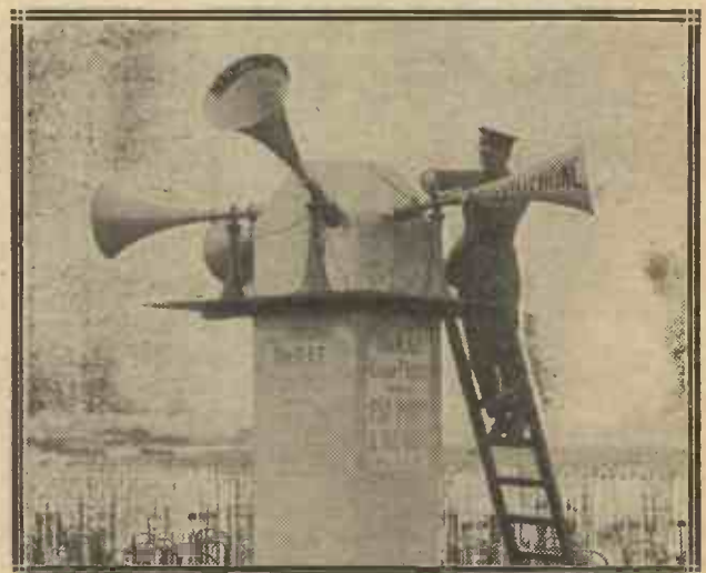
The powerful loud-speakers which were placed at intervals round the enclosures were linked to the main control room by means of buried cables.
