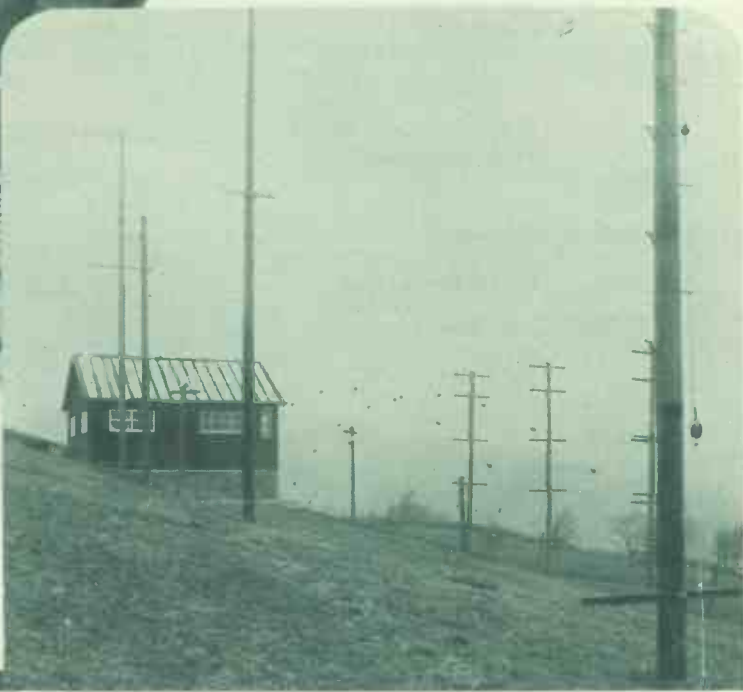
The ultra-short-wave aerial system at the G.P.O. station near Belfast, which is used for many of the ordinary telephone trunk calls between Northern Ireland and Scotland.
