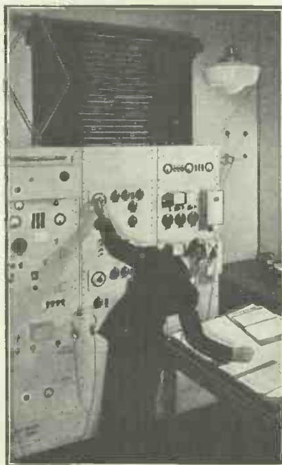
The direction finding panels in the B.B.C. check station at Tatsfield. You probably heard the broadcast a short time ago from this room, when the wavelength of the London Regional was checked.
