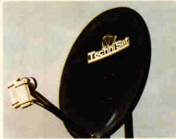
Fig. 1. One of the earliest dual- lnb satellite installations in the UK, as installed in December 1990. Both the original Marconi 1.3dB noise lnb s continue in daily use.
