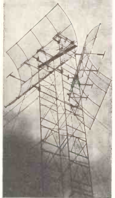
Typical TVR-1 repeater antenna installation.
