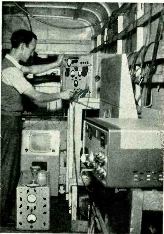
Interior of the transmitting van used at Harvel, near Wrotham. The technician is shown adjusting the gear associated with the S.T.C. microwave transmitter.
