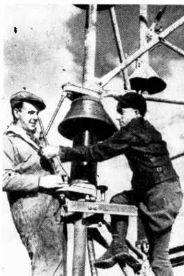
CHECKING INSULATORS on a 125-foot tower of one of the radio beacons which are being erected along the route of the trans-Canadian air line to Alaska.
