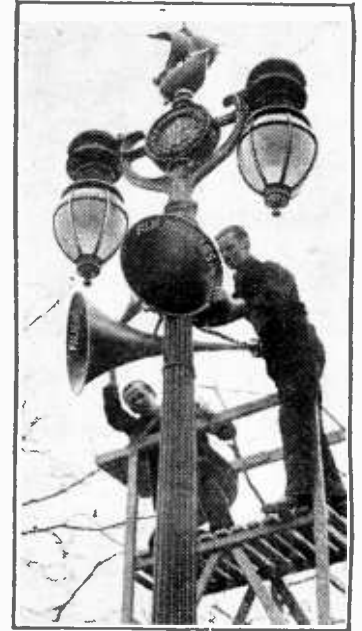
IN THE MALL. Film Industries speakers installed on a lamp standard.
