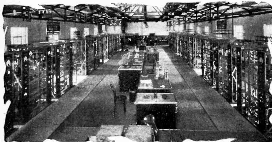
No fewer than eight Marconi beam transmitters are housed in this hall, from which direct communication is maintained with U.S.A., South America, Egypt, Japan and the Far East.
