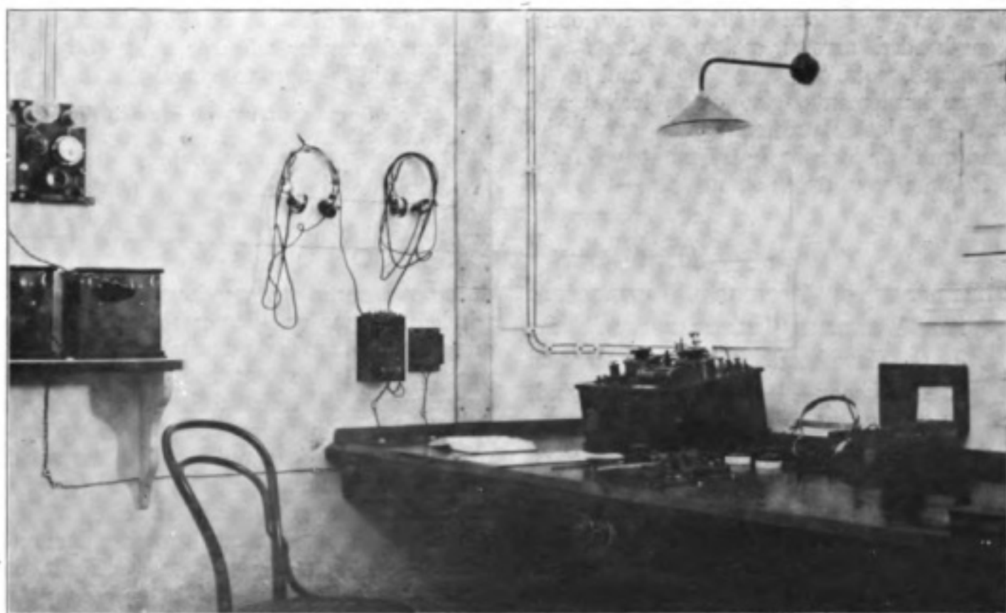
The Receiving Room of Antofagasta Station. From this room the transmitting apparatus is controlled by a system of remote control switches. The receiver used is the Fleming Valve, with necessary tuning condensers and inductances to render it responsive over very long range of wave length.
