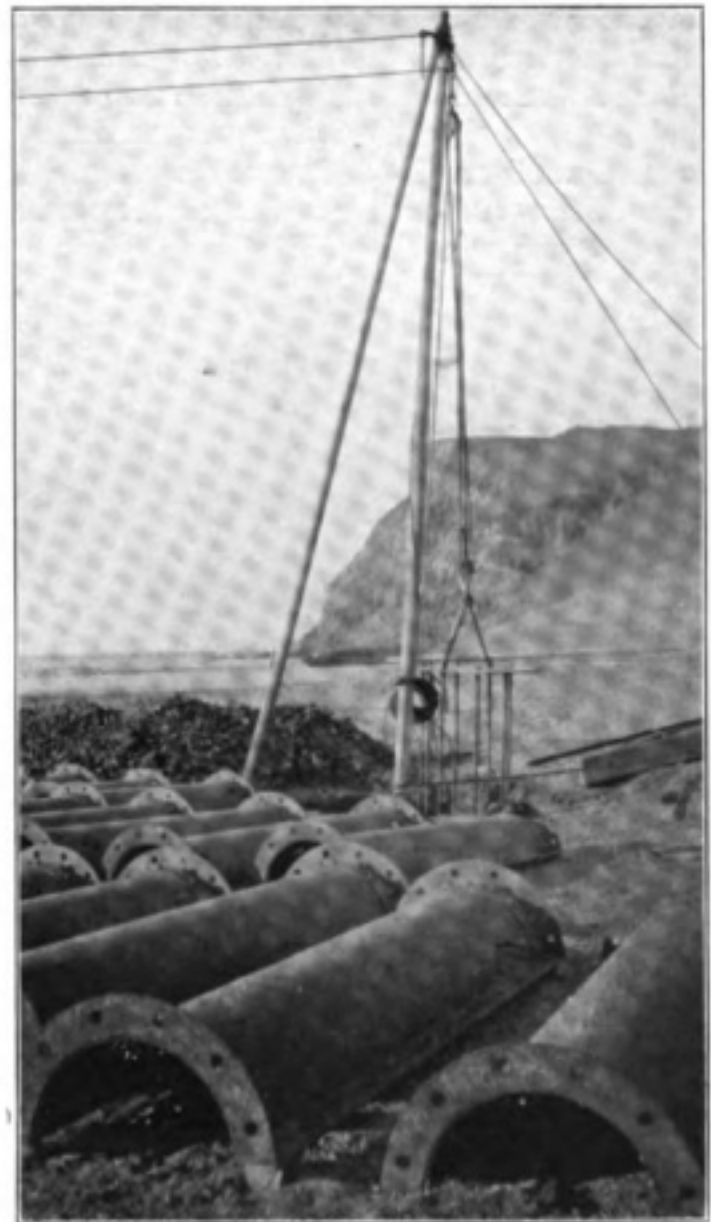
Lowering the base of the N.W. mast of the Arica Station into its pit. In the distance is seen the famous hill-fort, El Morro. The town of Arica lies immediately behind the hill.
