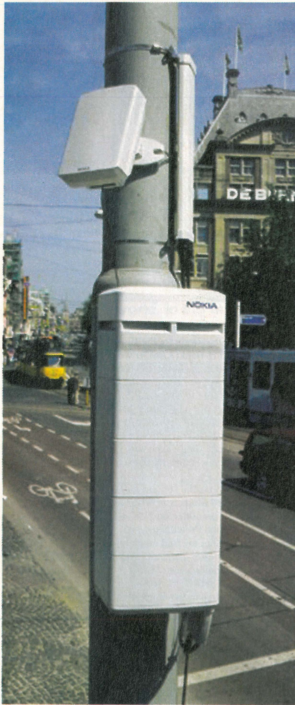
Typical streetworks base station site
