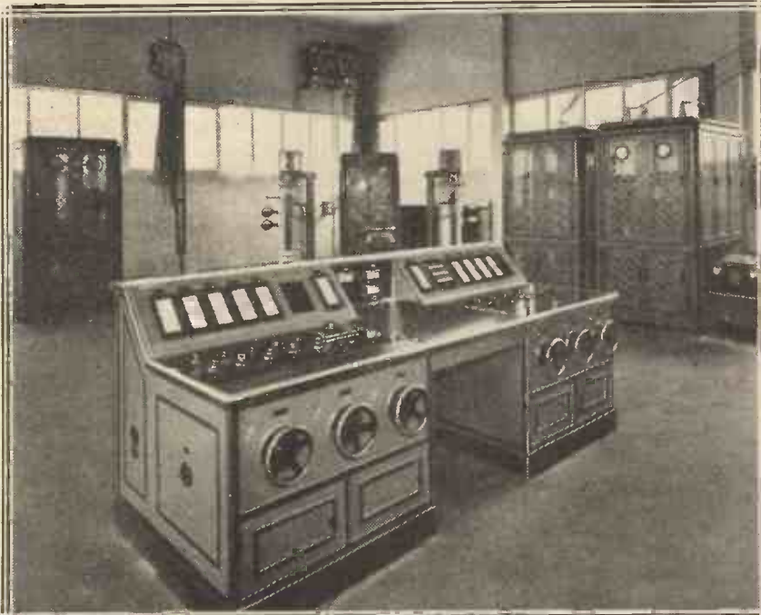
The imposing array of meters on the control desk at the Frankfurt station tells the engineer-in-charge exactly how the transmitter is working without his having to inspect each part of the apparatus.
